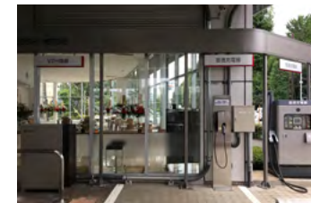
V2H and Charging Corner
