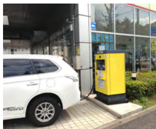
Quick charger installed in a dealer
