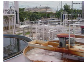
General effluent treatment facilities
