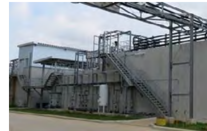
Industrial water/wastewater treatment plant (Far left: industrial water treatment plant, Right: Wastewater treatment plant)
