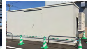
Storage battery unit
