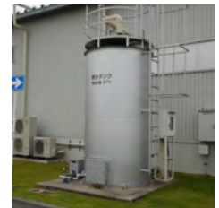
Rainwater storage tanks (Okazaki Plant)
