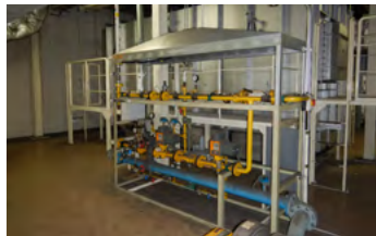
Deodorizing equipment for electrodeposition drying furnaces to reduce VOC emissions (Okazaki Plant)
