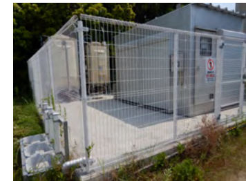
Groundwater membrane filtration equipment (Okazaki Plant)
