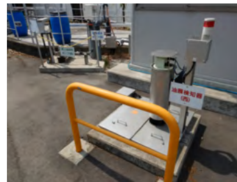
Surface oil detector (Okazaki Plant)
