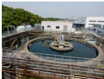
General effluent treatment facilities (Okazaki Plant)
