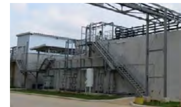
Industrial water and wastewater treatment plant
