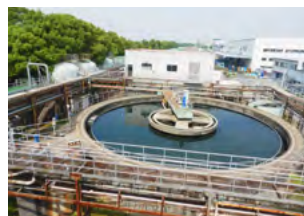
General effluent treatment facilities (Okazaki Plant)
