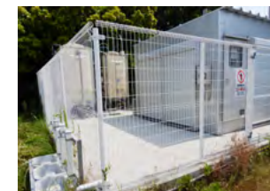
Groundwater membrane filtration equipment (Okazaki Plant)
