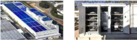
Solar power system and battery storage system installed at the Okazaki Plant (Aichi Prefecture)
