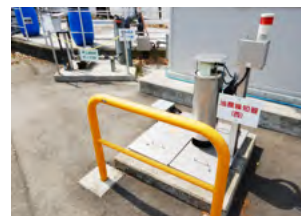
Surface oil detector (Okazaki Plant)
