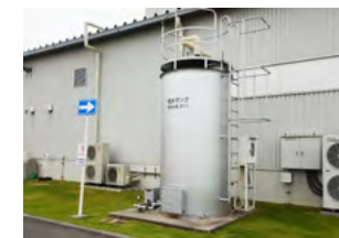
Rainwater storage tanks (Okazaki Plant)
