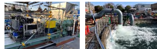
"DELICA D:5" engines driving drainage pumps
