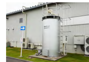
Rainwater storage tanks (Okazaki Plant)
